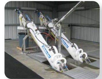
12 - Flo-Drum Units with Heat Tracing in Washington State
