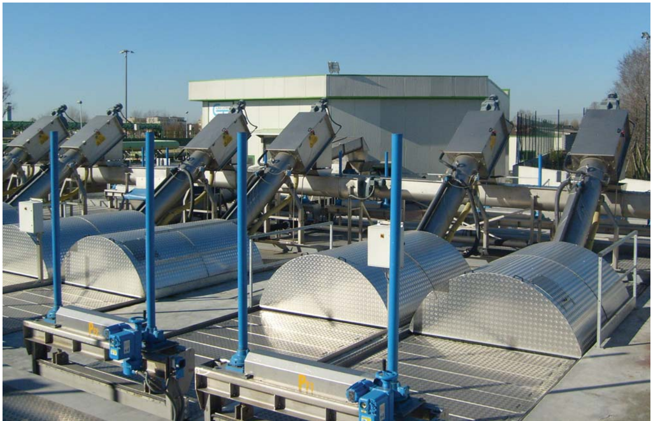
Six FD-MBR2000 10 MGD Per Screen - Brescia Italy
